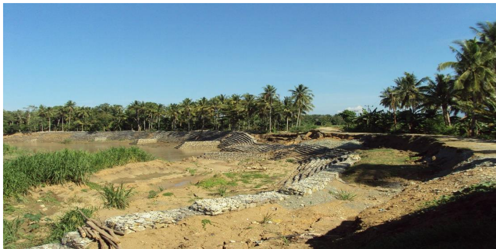
Figure 3. The appearance of subsidence on the road of the study location
